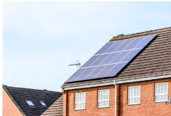
Photovoltaic panels generating electricity. Alternatively solar thermal roof panels can be used to generate hot water.
